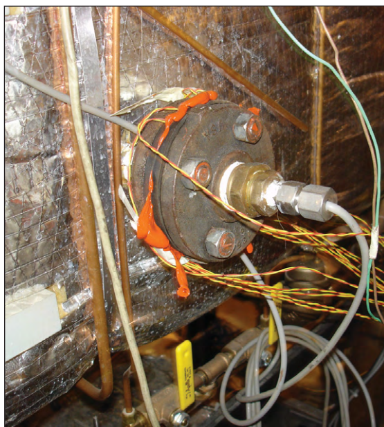
Figure 2 • Temperature-sensing wire is fed inside the chamber through a gasket gland.
